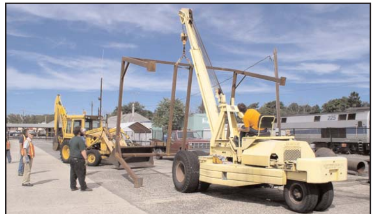
Randy Natale operates the crane while Justin Chapin and Dave Roberts look on as the new housing for the forge exhibit is turned upright.
