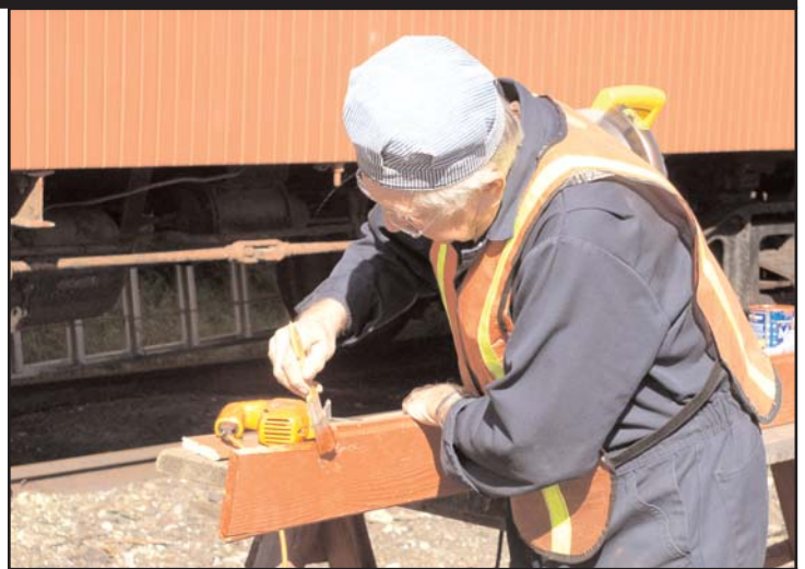
Volunteer Gerry Herrmann paints a new wooden panel that will replace a rotted one removed from the NYCHRR caboose #19322 currently being restored.
